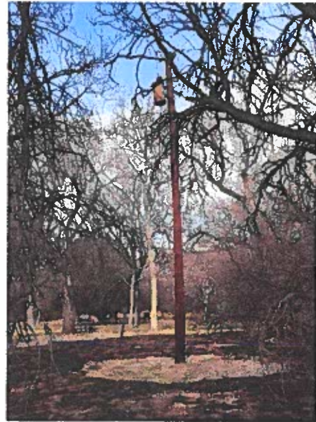
Example of Defensible Space Around Poles
